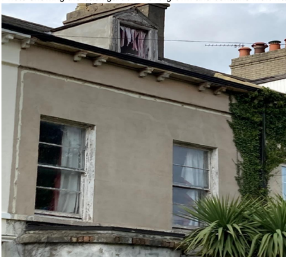
Photo showing the top window missing – pigeons entering this room
