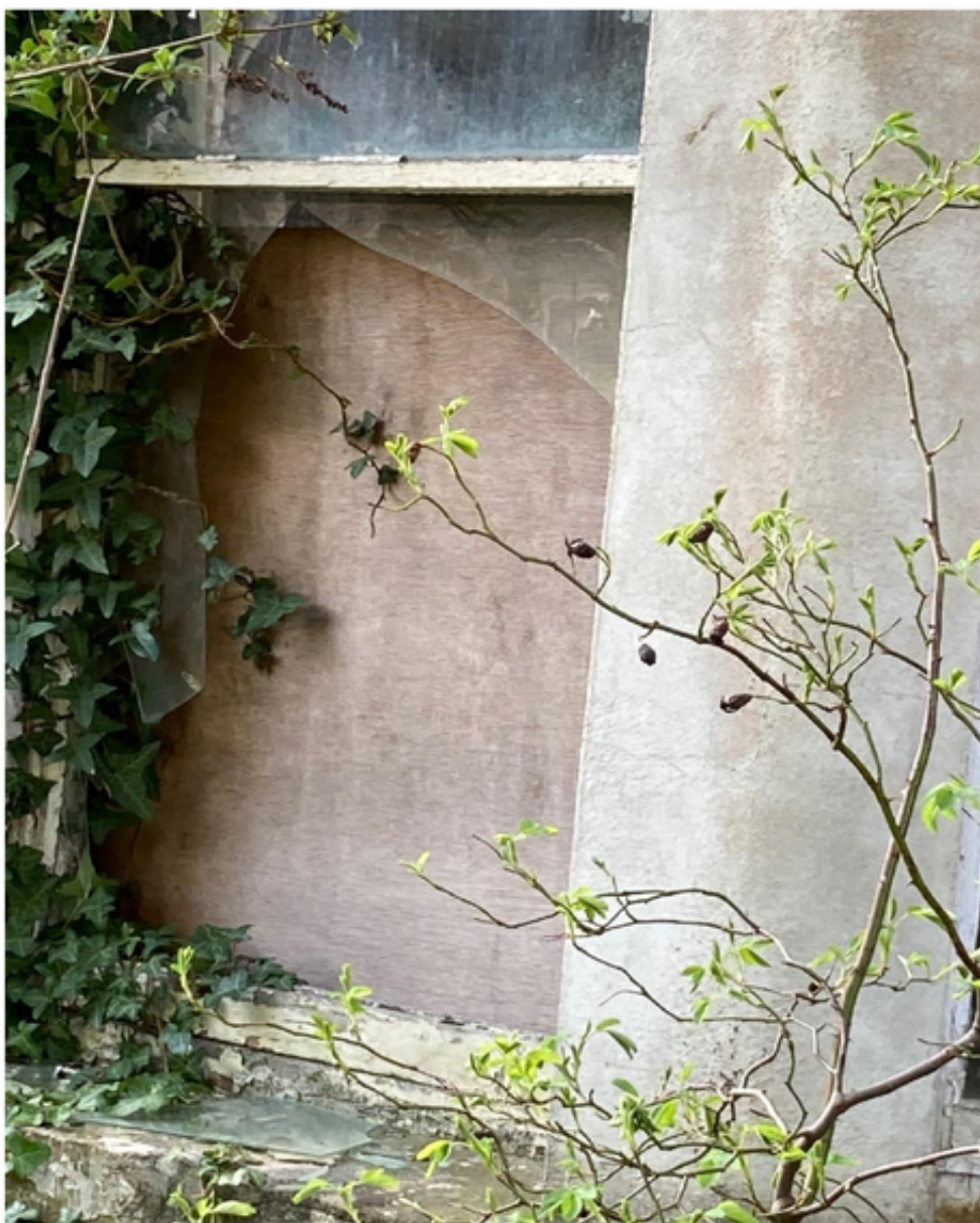
Photo showing front living room window – missing windowpane and sheet of plywood propped against it.
