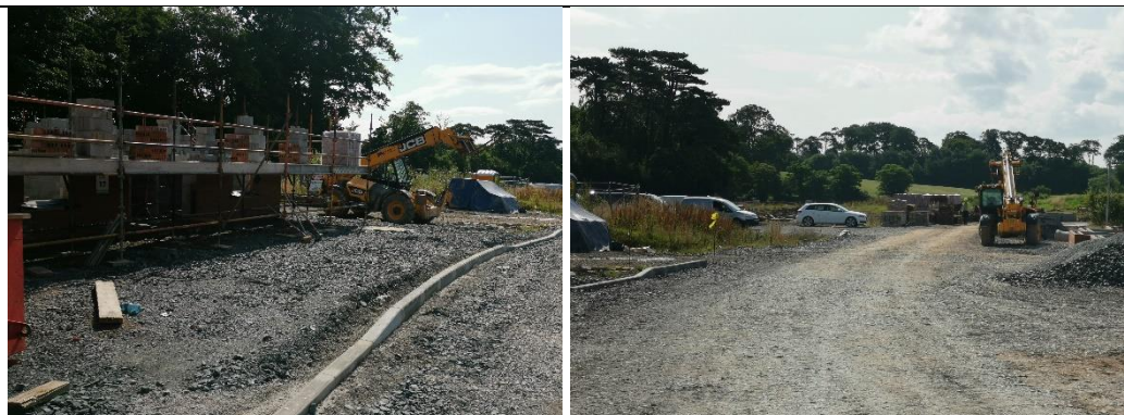
Photos 4 & 5: Views towards application site with adjacent dwelling no17 under construction (left)
