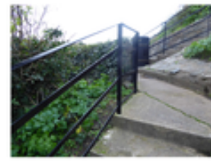
New handrails to steps (as noted) to match existing estate type railings
