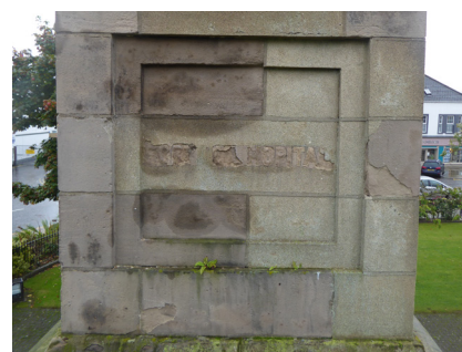
Fig.13 - Loss of raised lettering
