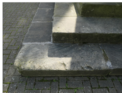
Fig.05 - Delamination to steps
