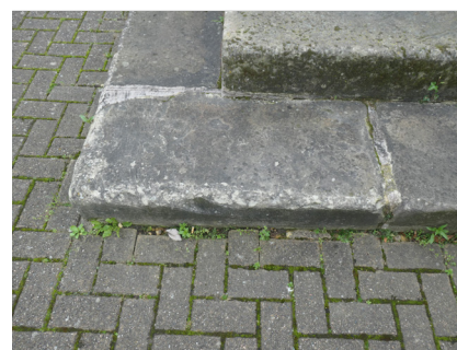
Fig.18 - Spalled edging to steps
