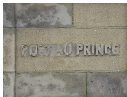
Fig.25 - Partial loss of lettering
