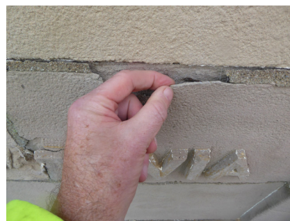
Fig.33 - Advanced decay of stone
