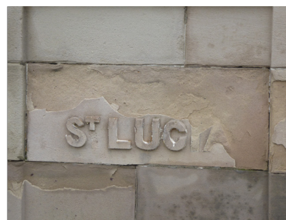
Fig.22 - Partial loss of lettering
