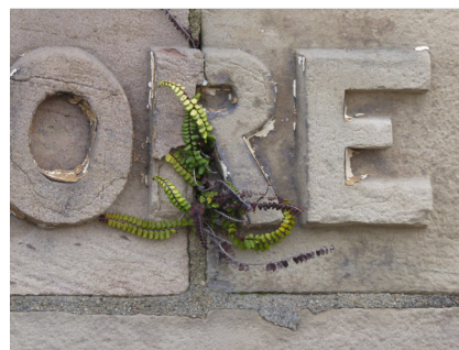
Fig.43 - Open joints with light vegetation
