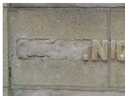
Fig.36 - Loss of raised lettering
