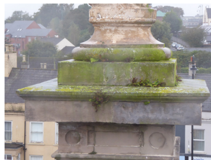
Fig.37 - Heavy algae staining
