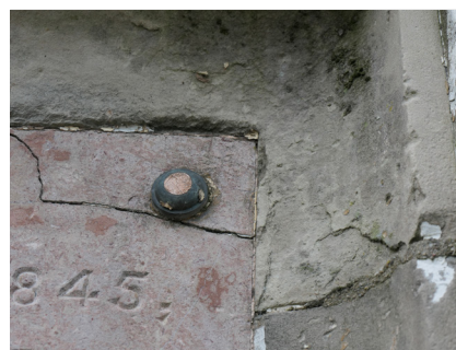
Fig.31 - Fracture on limestone tablet
