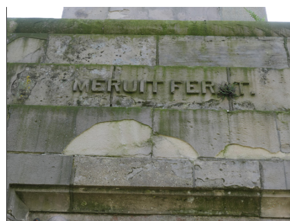
Fig.08 - Contour scaled delamination
