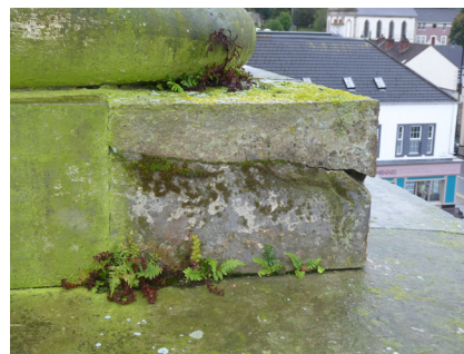
Fig.15 - Heavily fractured stone
