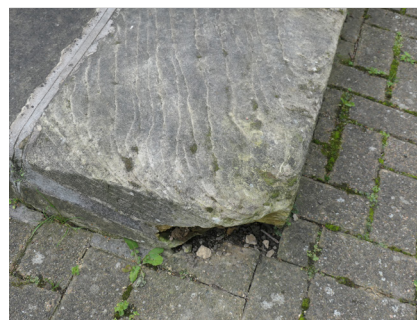
Fig.28 - Advanced decay of stone step
