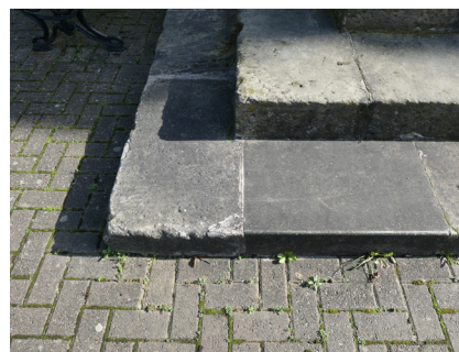
Fig.38 - Spalled edging to steps
