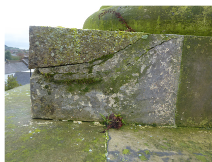
Fig.46 Heavily fractured stone
