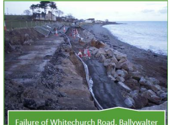
Failure of Whitechurch Road, Ballywalter due to coastal erosion (source DfI Roads)
