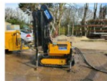
See My notes for plan to avoid damage to existing structures
