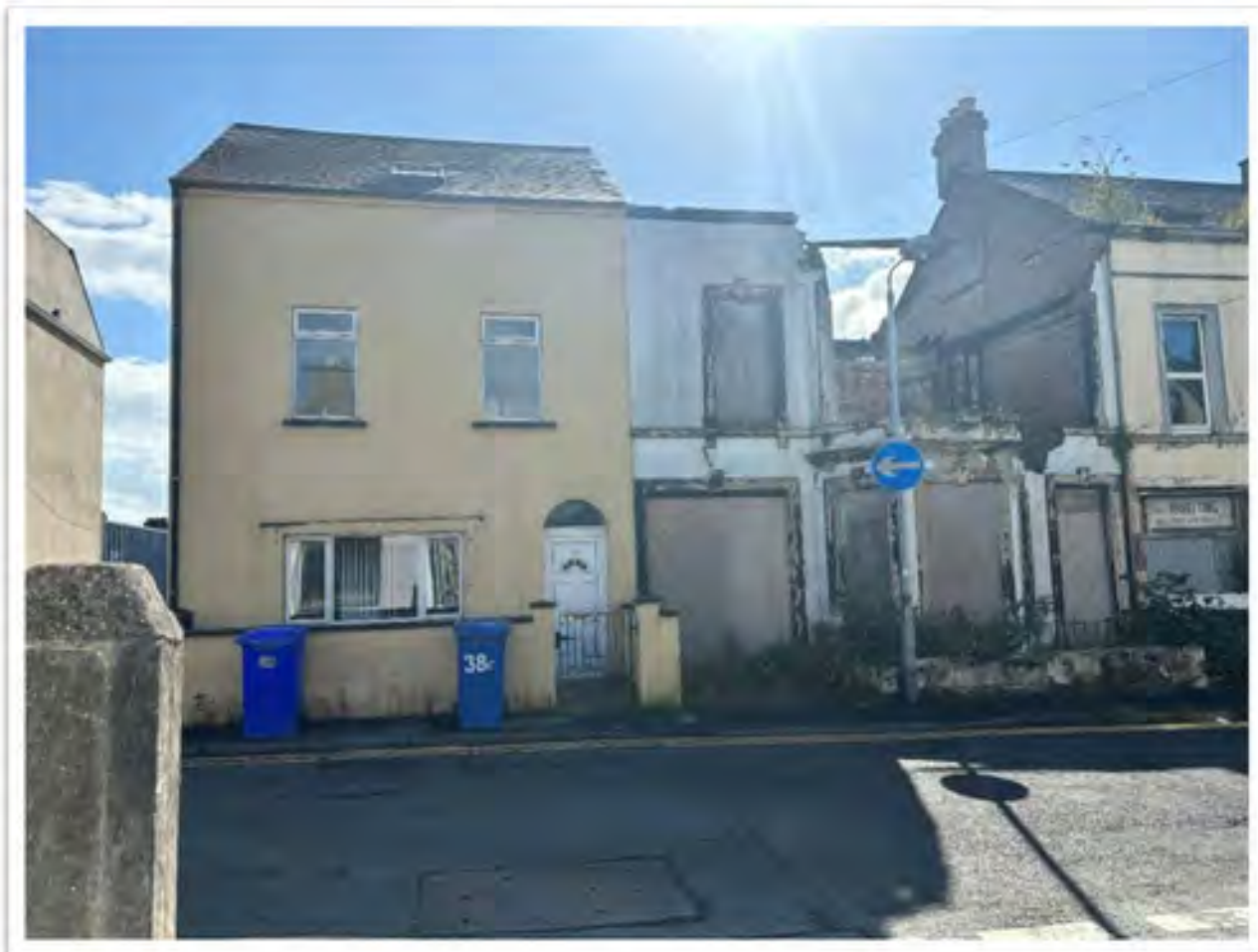
Figure 3: Existing Site Frontage, showing extensively fire damaged dwelling in centre of terrace
